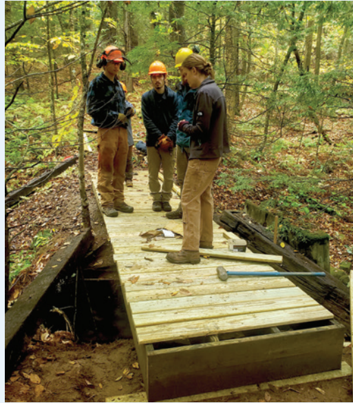
Four new bridges over streams and ravines at the 40-acre Annie Sturgis Sanctuary in Vassalboro, ME, were completed late last spring. The work came at an ideal time for people seeking the solace of nature to enjoy safely distanced walks at this state-listed Critical Natural Area.
